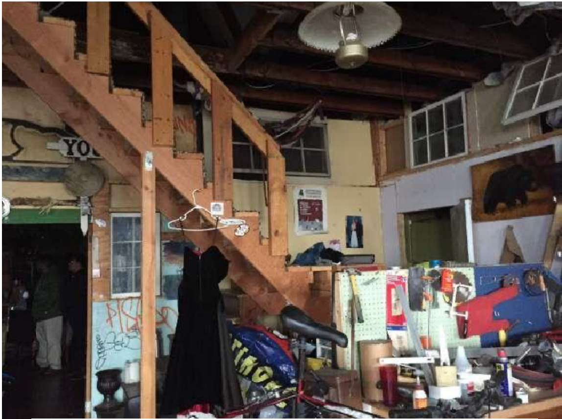
Figure 7: This Dec. 6th 2016 photo shows the interior of The Bell Foundry in Baltimore. Baltimore officials shut down the arts building Monday Dec 5th 2016 for safety violations and evicted dozens of tenants three days after a fire at a California warehouse-turned artist enclave killed three dozen people (Linderman 2016)
