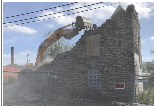
CREWS RIP DOWN HISTORIC STONE HOUSES IN BALTIMORE'S WOODBERRY NEIGHBORHOOD. (FRED SCHARMEN)
